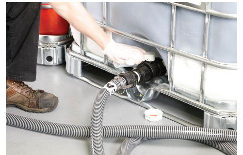
24) Shut off both tote valves and turn off at the main power source.
