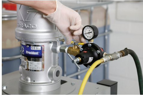
14) Turn the air supply to the air motor pump on.
